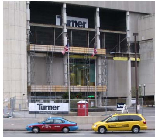
Precision planning and execution led to successful removal of precast panels above the existing glass curtain wall.
