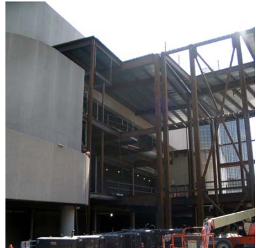
Double columns signify the separation between the bridge deck construction and expansion of the existing building structure.
