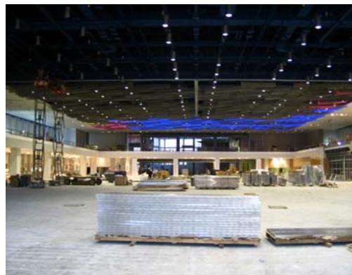
Pattern drawn on ballroom floor provided for accurate installation of the 1,250 lighted ceiling fins.
